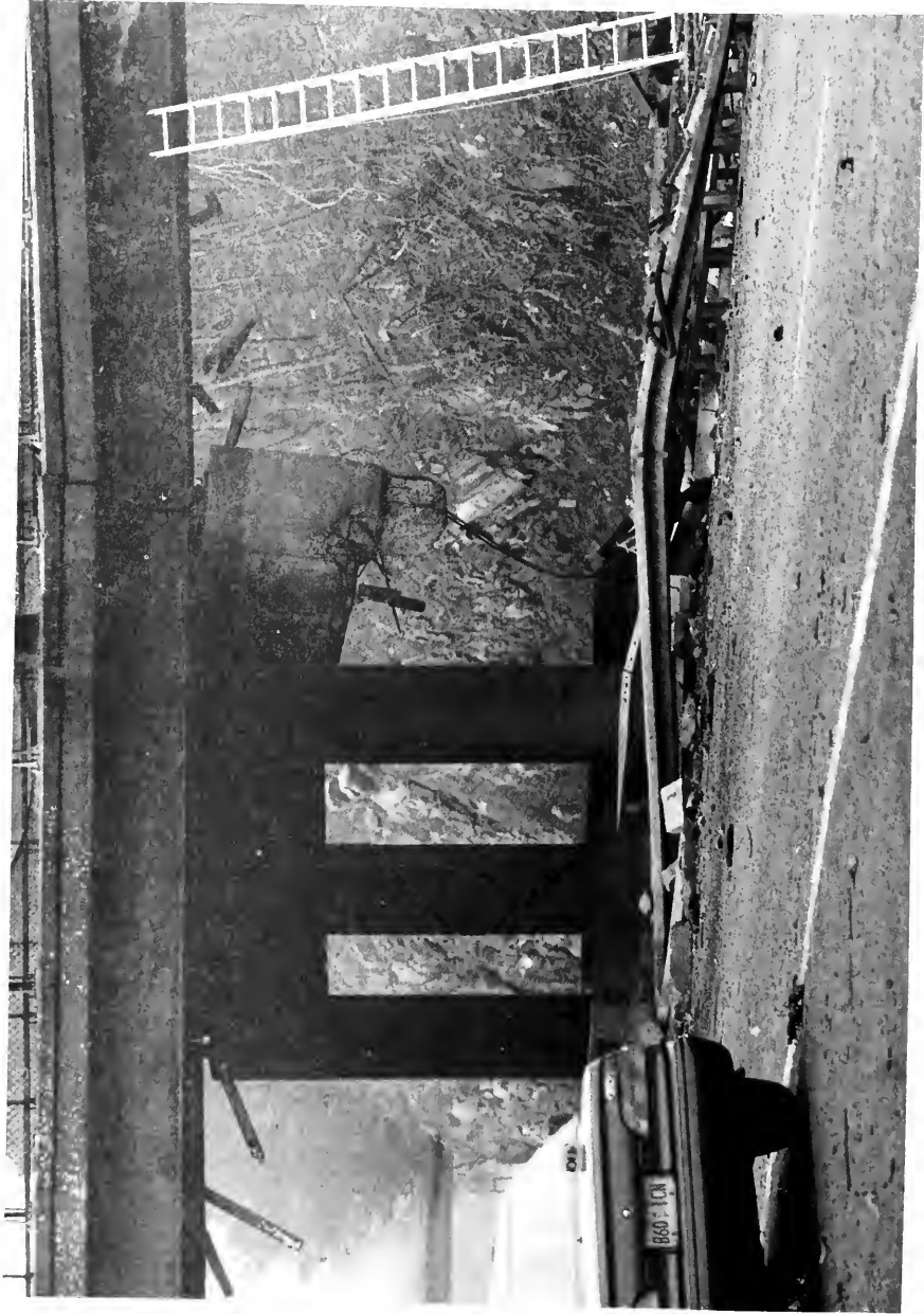
Figure 6. -- Damaged column of Grant Avenue overpass (Photo by Mike Horn)
